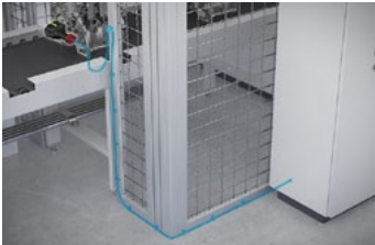
No need to spend time on wiring
